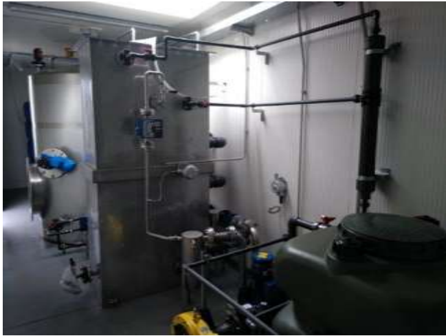
Anaerobic membrane bioreactor
