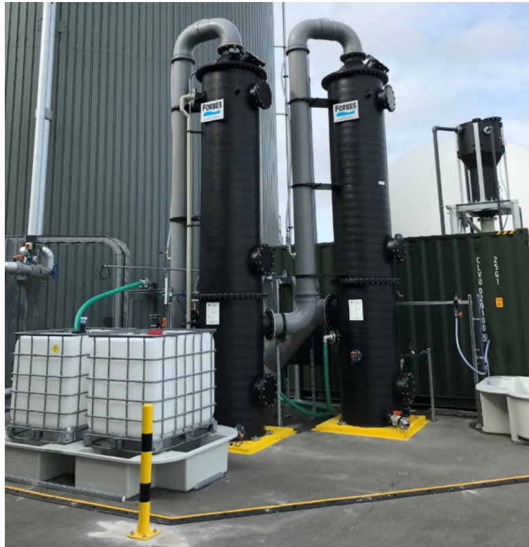
Figure 105. Ammonia stripping/scrubbing unit.
