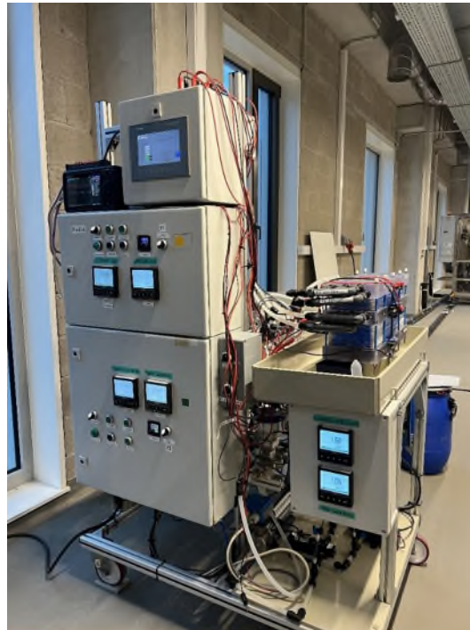
Figure 21. ED pilot installation.
