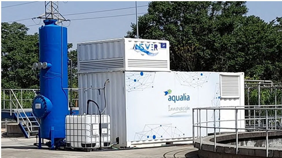
Figure 69. Picture of the ELSAR® pilot plant.
