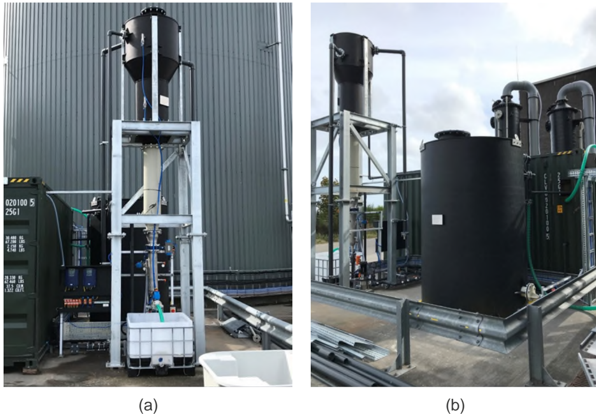
Figure 104. Struvite precipitation unit ((a) precipitation reactor and (b) clarifier).
