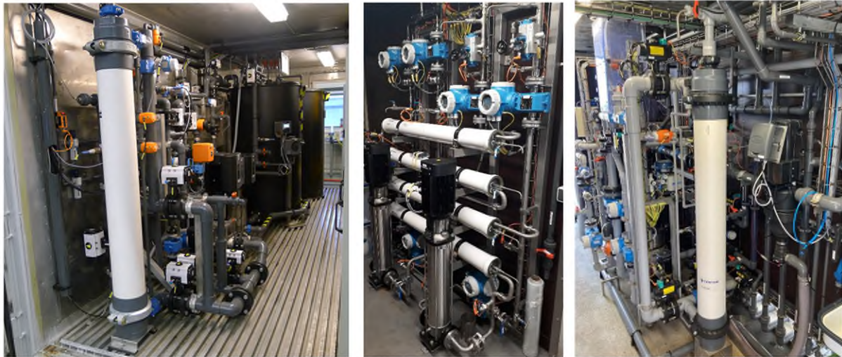
Figure 125. Pilot A - left: conventional ultrafiltration module; Pilot B - middle: reverse osmosis units and right: novel UF/NF module.
