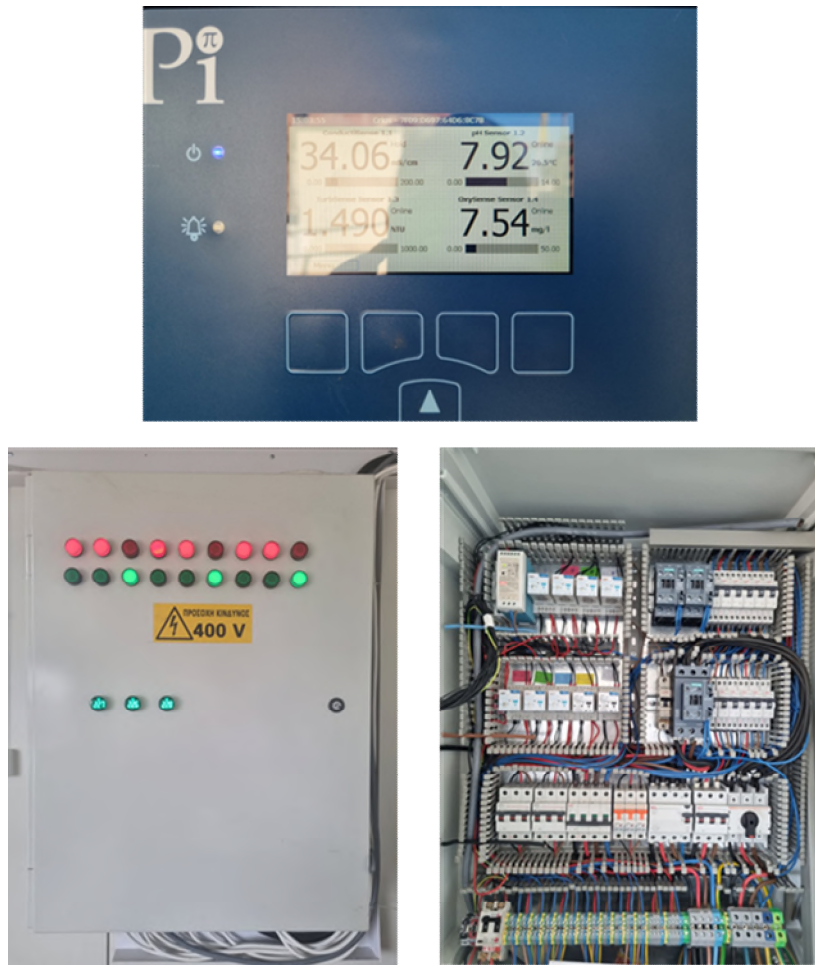
Figure 49. CS4 pilot plant sensors, control unit and TOC analyzer.
